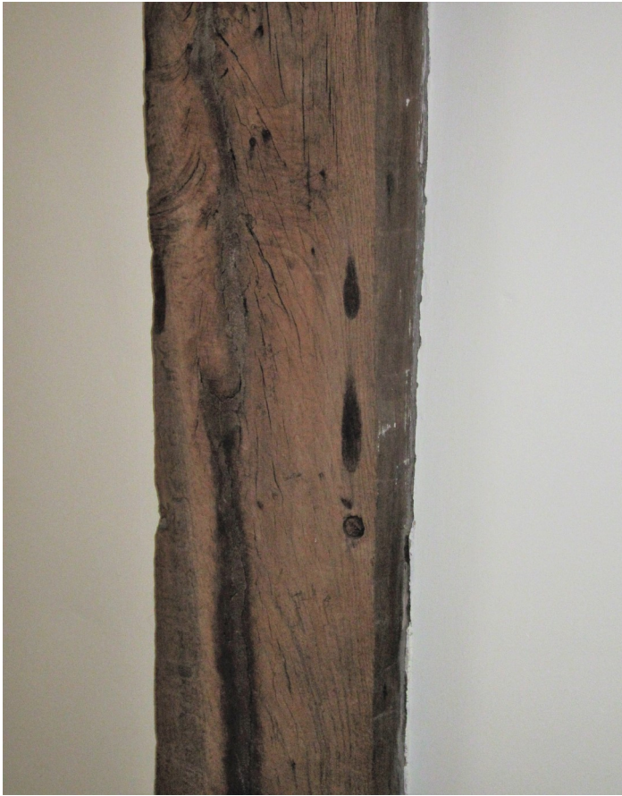
Lower Mill rear structure principle post scorch mark
